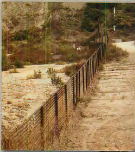
(left to right) PSP metal fence in Smuggler's Gulch. Note that to left (Mexico) side, ground level rises to top of fence. This entire section is watched by one USBP agent. Photo: Robert Burns
